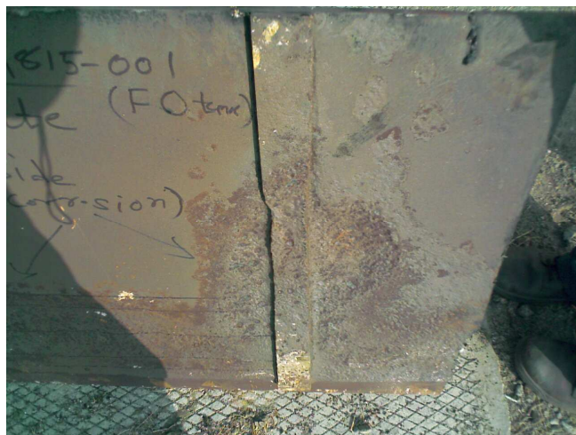
Soil Side Corrosion
