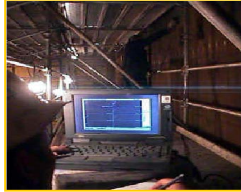
Waveforms are observed on line
